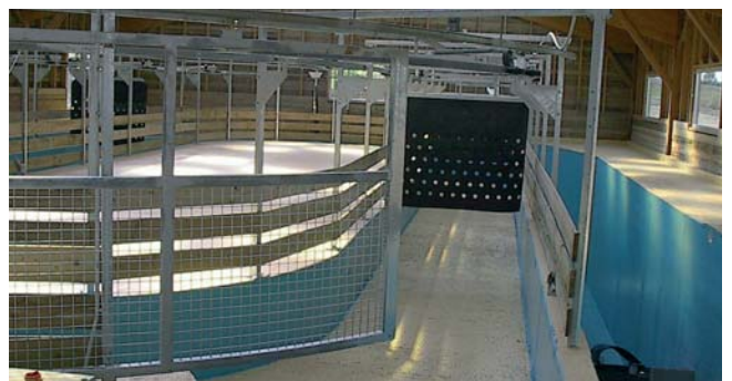
Rail-Gliding Horse Walker, Oval 10 x 20m (33'x66') for 6 horses installed in an existing building with pool, Haras de Sassy, St. Christop, France
